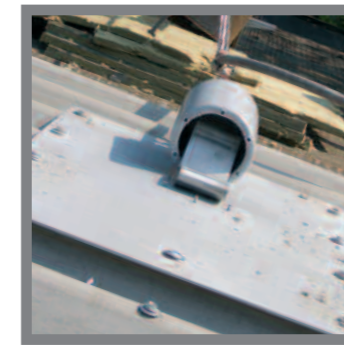
testing the system
